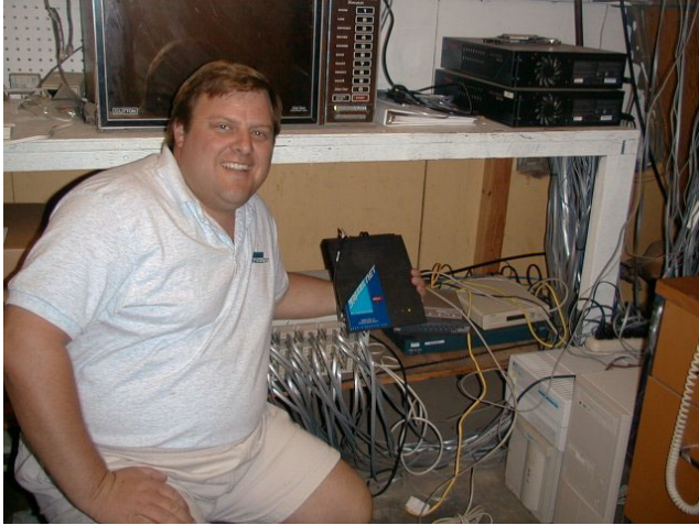
Marlon Shafer at Odessa Office Equipment’s Primary Point of Presence (POP) in downtown Odessa. Marlon is holding a BreezeCOM radio that’s used as a point-to-point link to a hub site located on a nearby hill.
